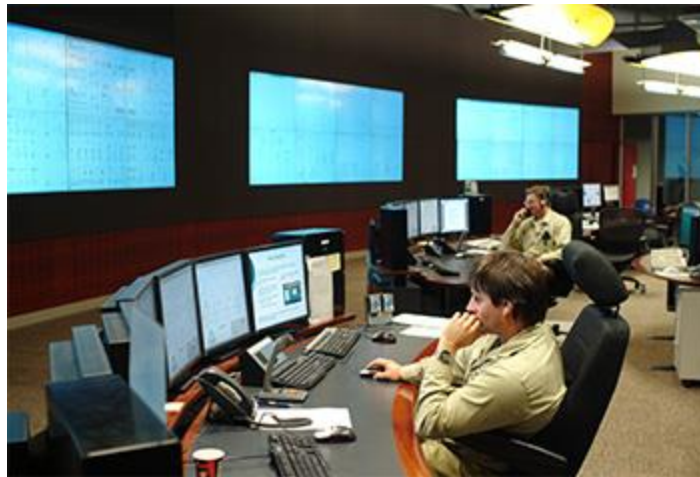
Process control room
